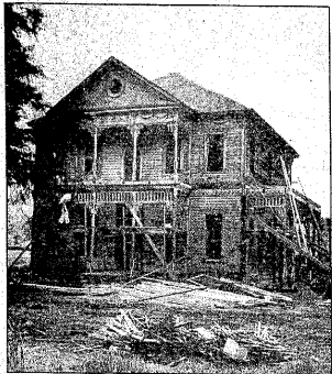
Auburn's threatened Neely Mansion.
